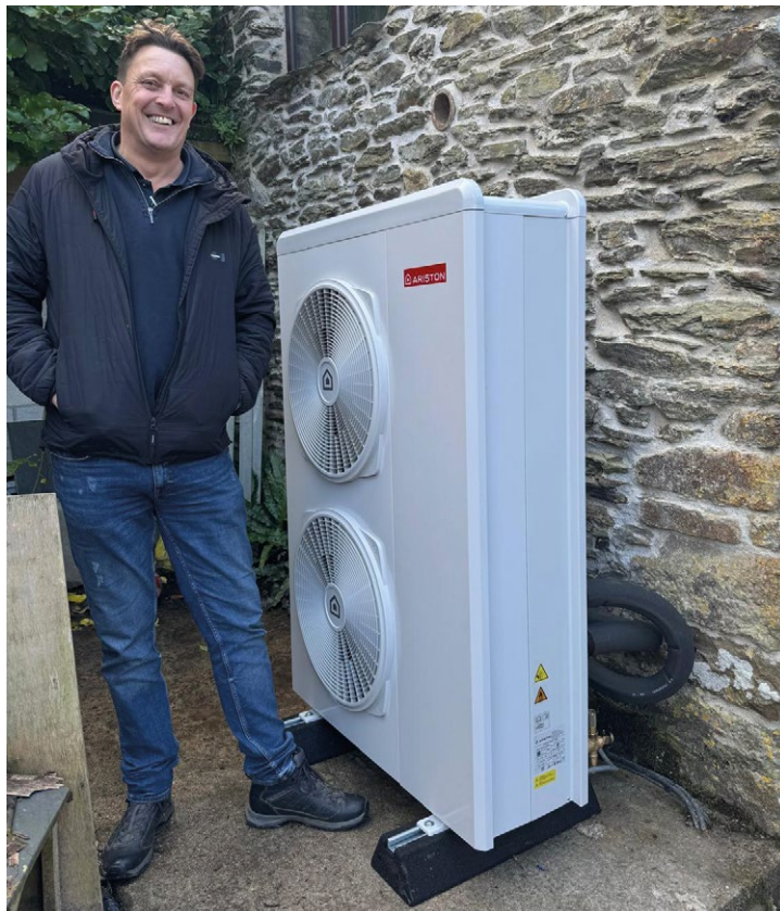
Terry Green (Homeowner) pictured with his new Ariston heat pump
